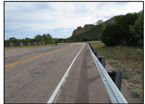
Recent local upgrades by CDOT include a wider shoulder and guardrail between La Veta and Cuchara.
