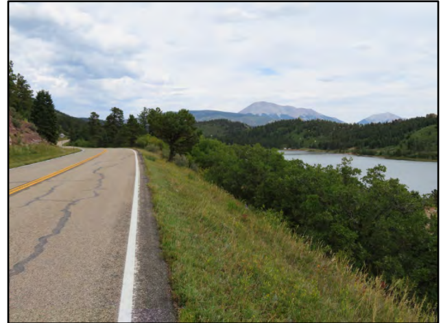
The byway roadway is characterized by steep grades, sharp curves, narrow shoulders and a limited roadside within the Alpine Segment.
